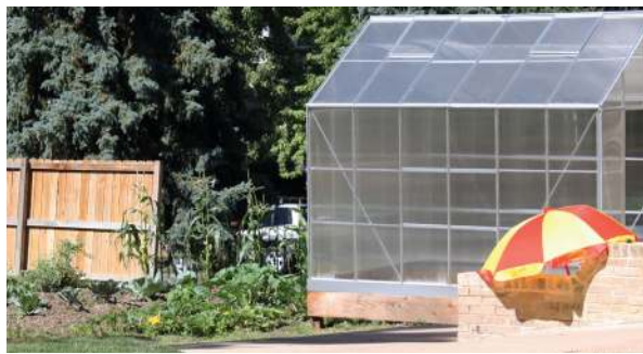
A new greenhouse has been added to our backyard vegetable garden! One of our AJJ members, Cynthia Haws, graciously donated the structure and the Rotary Club of Denver has been working on its construction.
